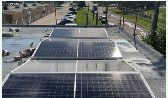
The Bee-Clean Edmonton office had 175 solar panels installed on its roof in 2023.
