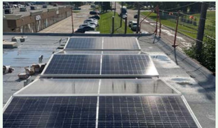
The Bee-Clean Edmonton office had 175 solar panels installed on its roof in 2023.
